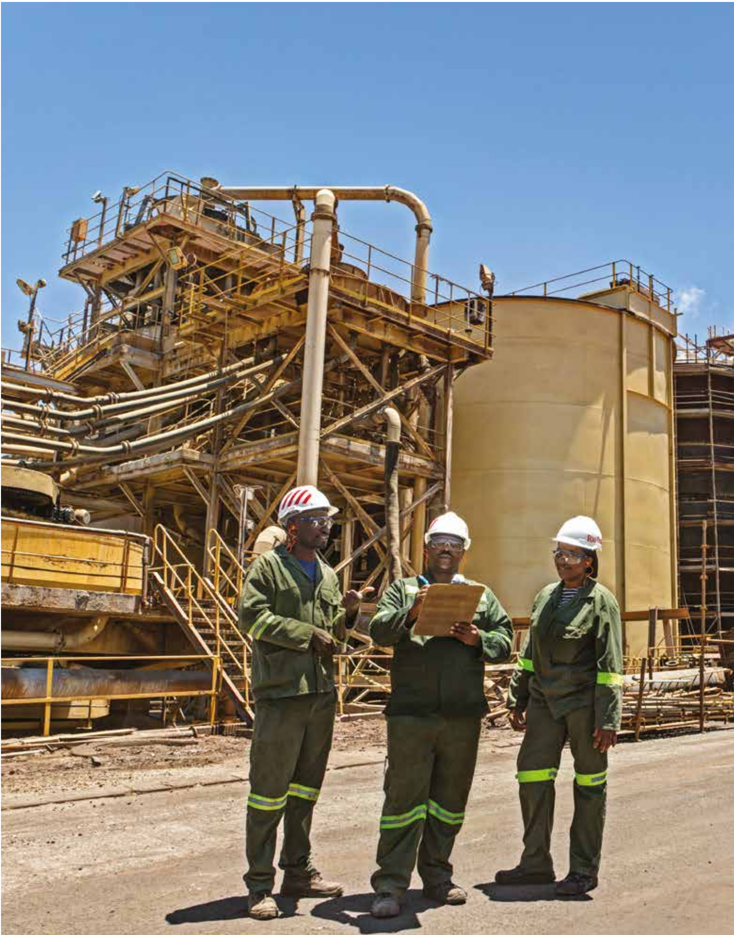
The refurbishment of the leach tanks is part of a ten-yearly refurbishment programme to ensure that the structure of the leach tanks is in good condition. Risk assessments are carried out by the workers to check that the work is carried out safely. Employees of the Namibian Engineering Corporation (NEC), Sam Nujoma, Stephanus Mouton and Teopolina Fanuel are conducting a safety check while working on the refurbishment of one of the leach tanks.
